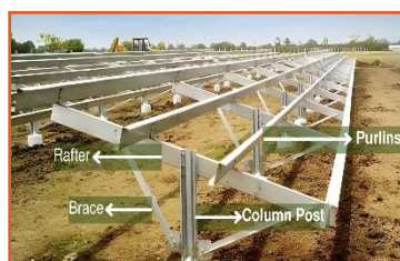
Fixed Tilt Structures
