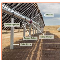
Solar Tracker Structures
