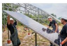
Solar module mounting structures Fixed-tilt frames; 113,000 MTPA (~6.28 GW)
